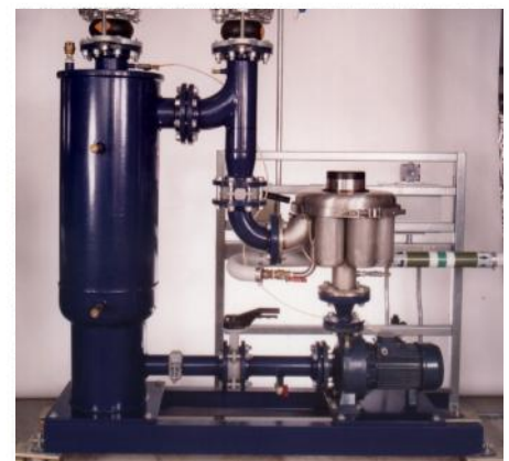
4 Forced Sedimentation System – Phoenix
