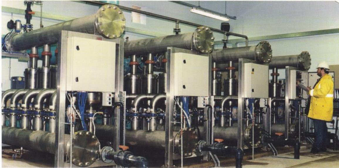
Four banks of System 2000 filters installed in a water treatment works.
